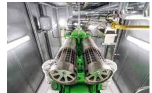
GENERATOR IN CHP PLANT
